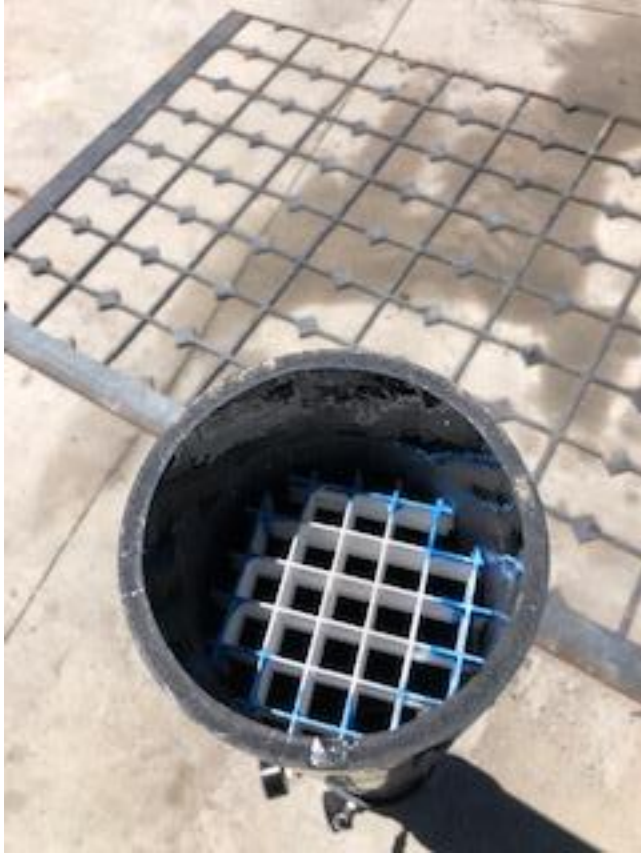
Figure 6 Flow straightener grid in inlet of Pitot Tube Flowmeter
